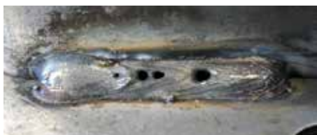
Fillet weld with pores: Real image
